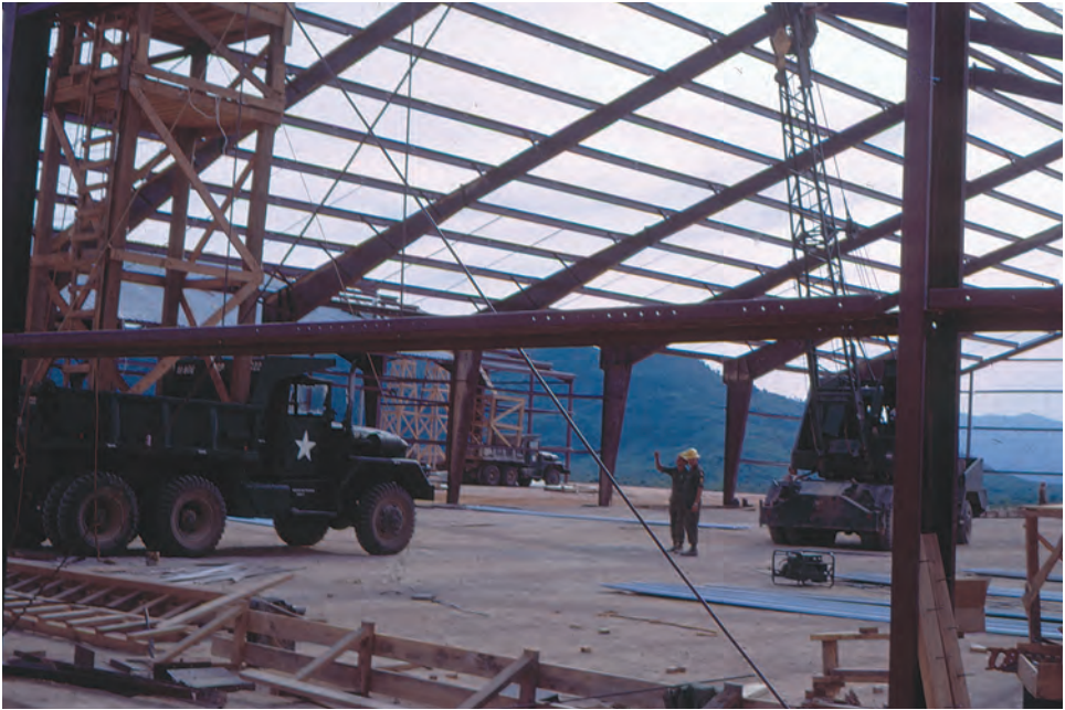
In 1967, construction of depot facilities outside Qui Nhon were under way such as this Butler warehouse building being built by the 19th Engineer Battalion at Long My.
